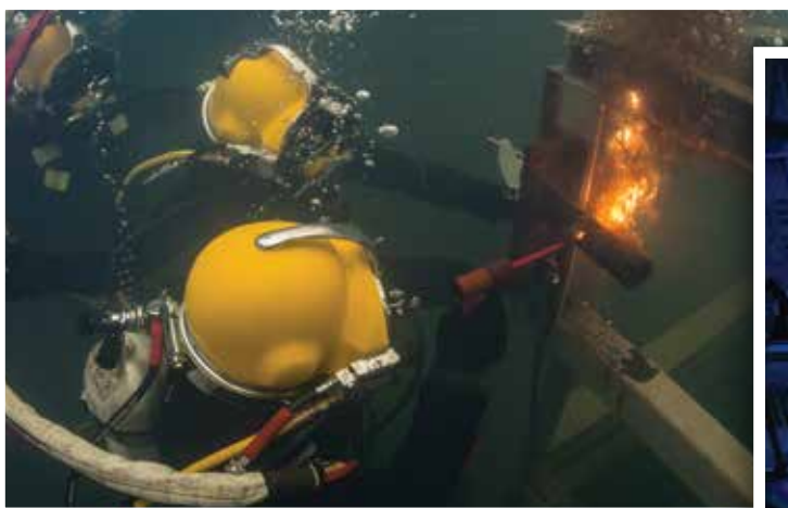
ABOVE: A member of the ROK Navy's Underwater Construction Team practices underwater cutting techniques with Sailors during exercise FOAL EAGLE at the ROK Naval Education and Training Command in Jinhae, Mar. 31, 2017.
